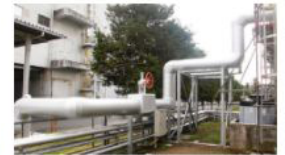
Steam emitted from the Center is sent to the property of Hisamitsu Pharmaceutical.
